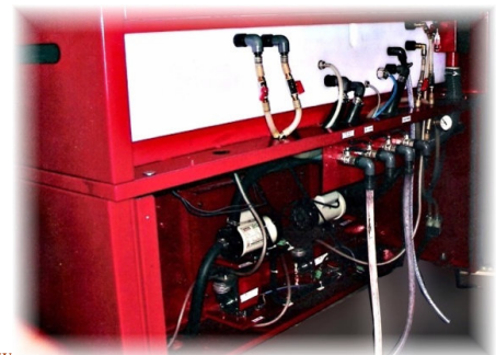
V P X Plumbing Side View
